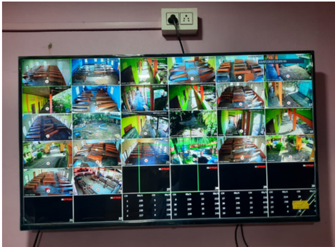
CCTV surveillance (College Campus)
