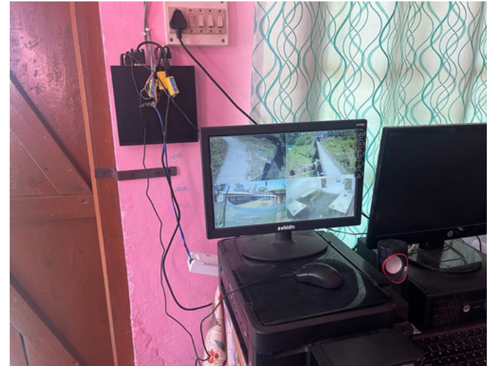
CCTV surveillance (Boys' Hostel)
